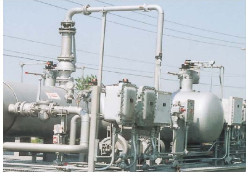
Mixing and Analyser system
